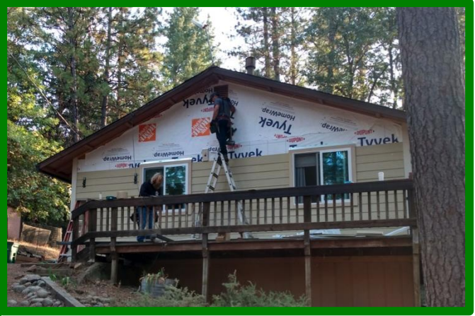
Homeowner installing fiber cement siding over old wood siding, Twitchell Rd area
